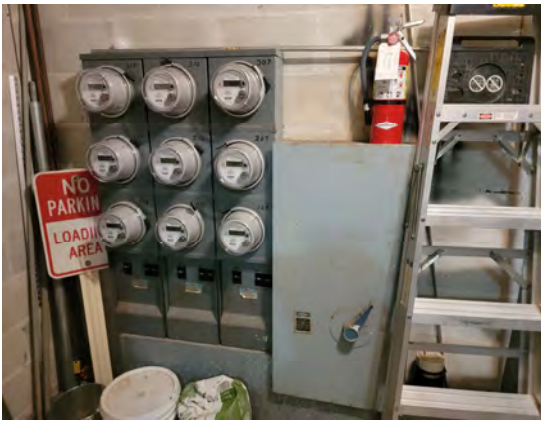
73 Meter Bank and Disconnect
