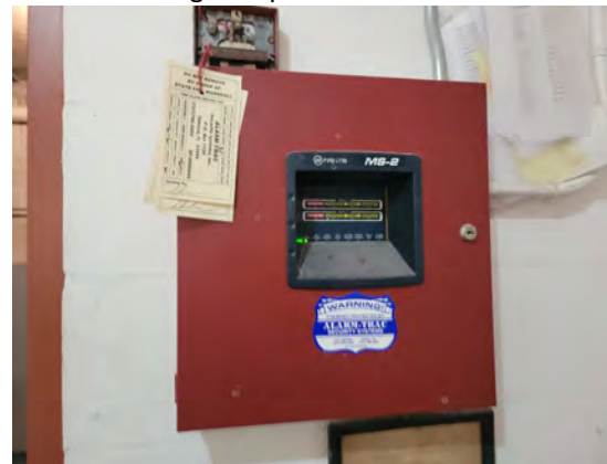
70 Fire Alarm Panel
