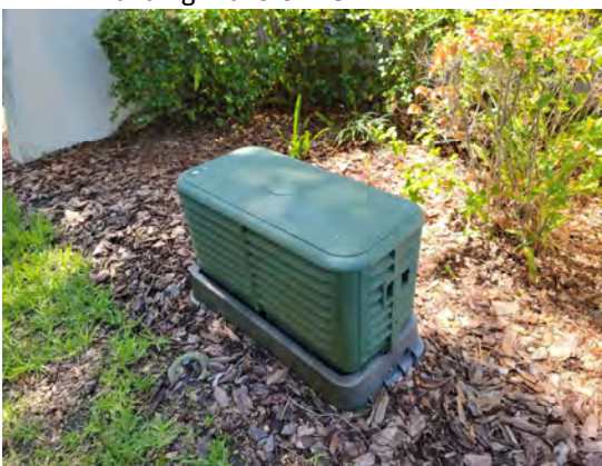
79 Cable Connection Box
