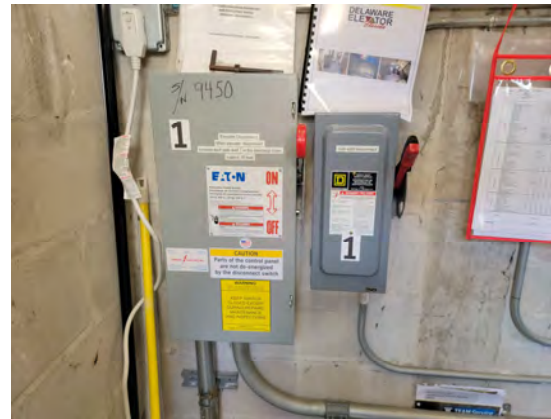
60 Elevator Electrical Disconnect
