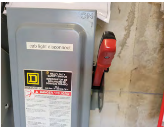
61 Elevator Lights Disconnect
