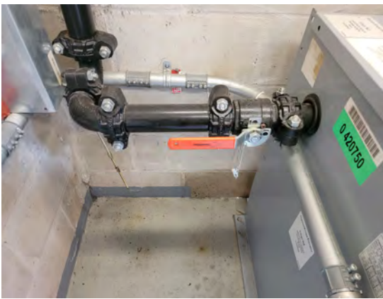
65 Elevator Pump Disconnect
