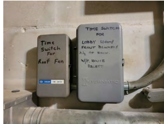
76 Electrical control Timers for Roof Fan
