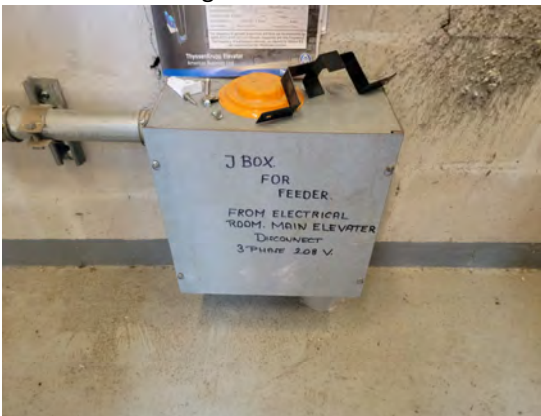
63 Elevator Junction Box
