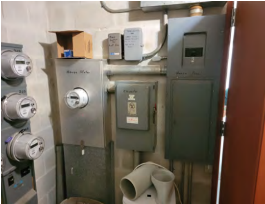
75 Meter Bank and Disconnect
