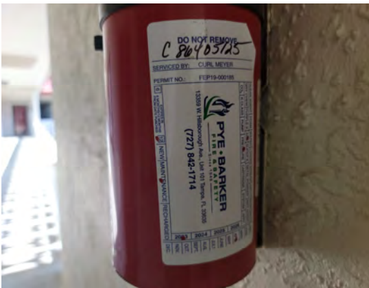
45 Fire Extinguisher Data Label
