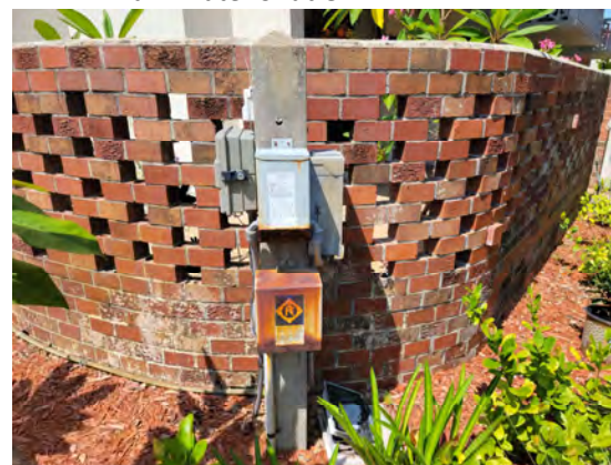
80 Electrical Timer Boxes
