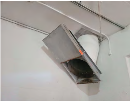
69 Trash Chute Above Dumpster
