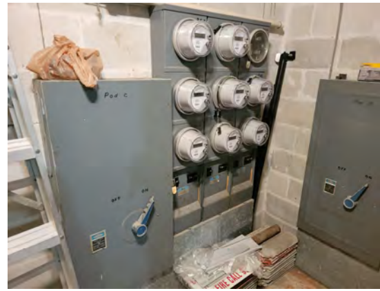
74 Meter Bank and Disconnect
