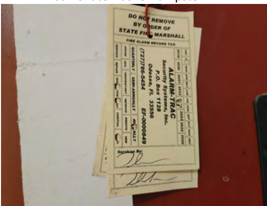
71 Fire Alarm Data Label
