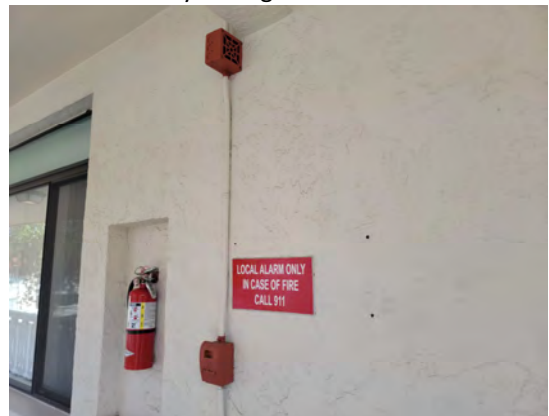
48 Fire Alarm Pull Block
