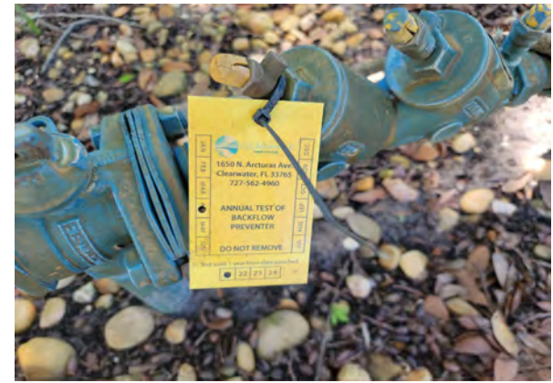
14 Backflow Valve Data Label
