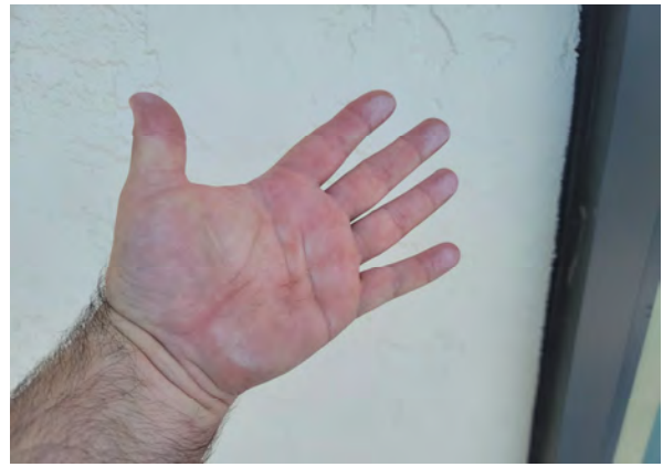
26 Exterior Paint Chalking
