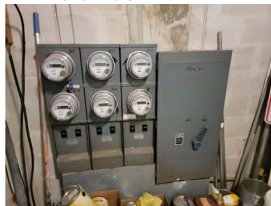
72 Meter Bank and Disconnect
